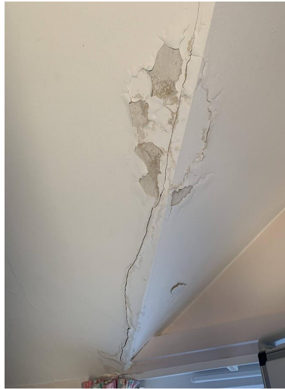
Example of roof issues
