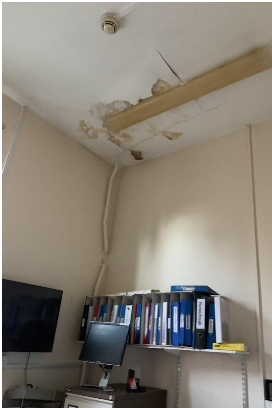
Internal damage from issues with pitched roof
