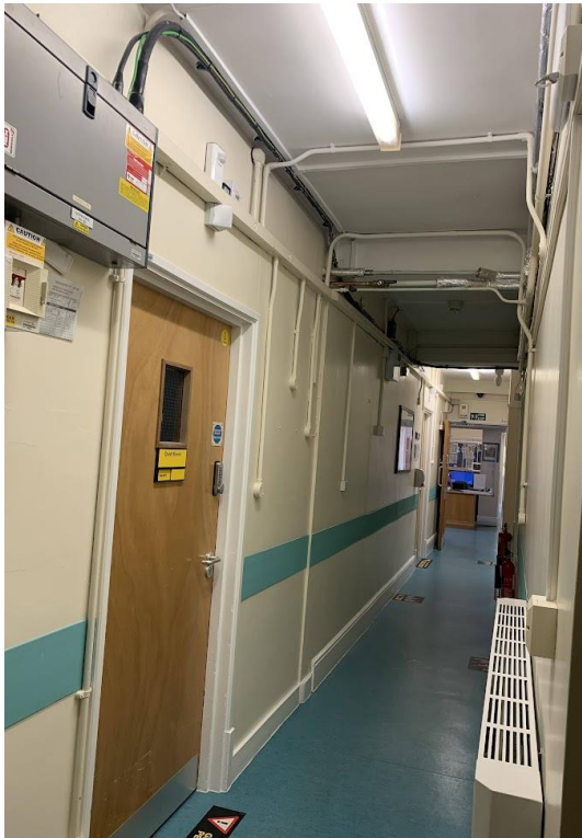
Example of infrastructure in ward corridor
