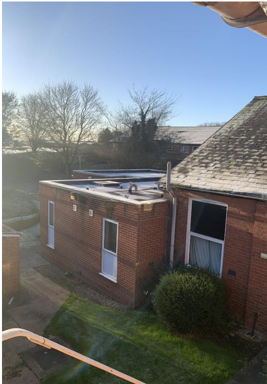
Example of problematic roof and only fire exit
