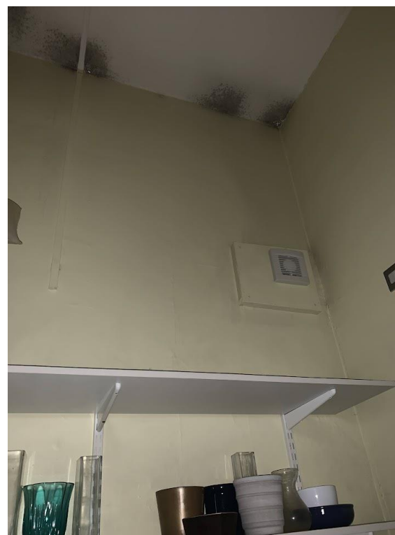
Dirty utility only ventilation
