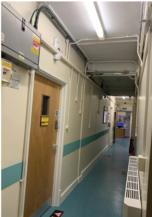
Example of infrastructure in ward corridor
