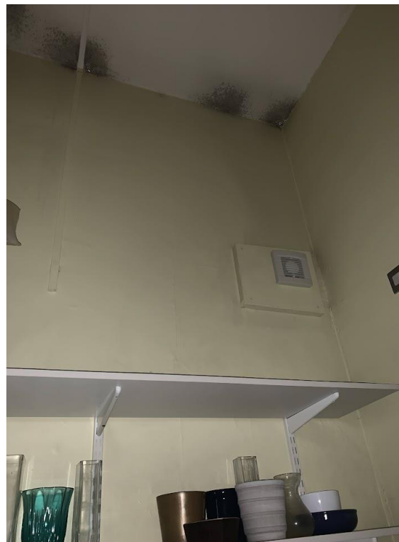
Dirty utility only ventilation
