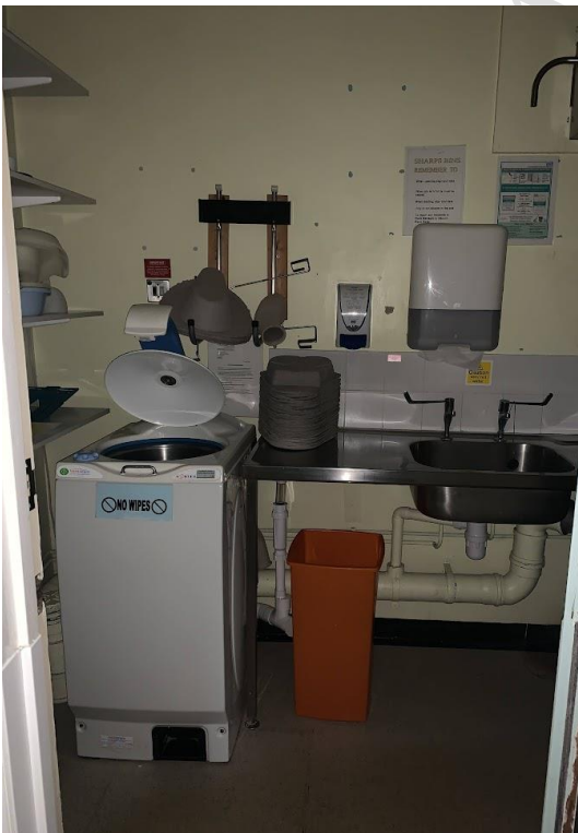
'Dirty' utility and no 'clean' area
