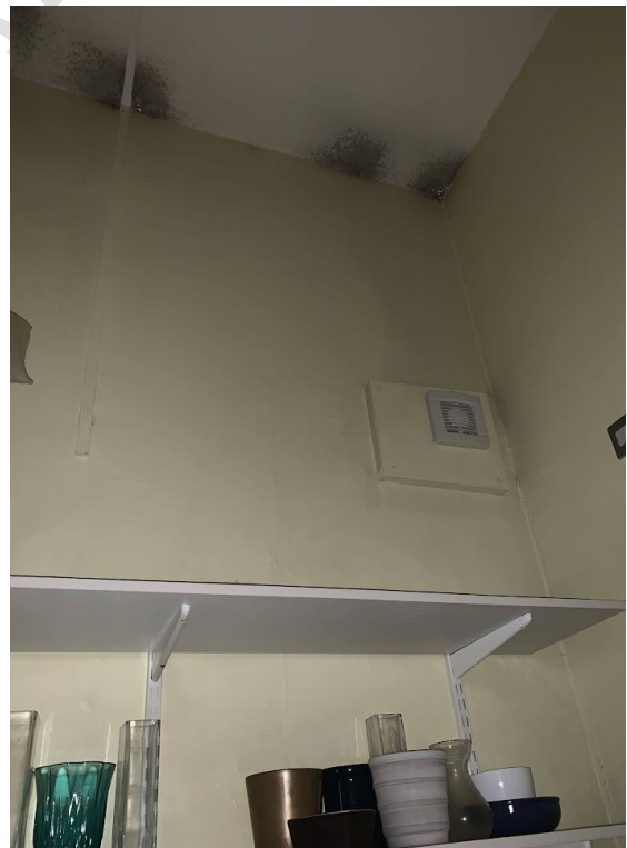
Inadequate ventilation for a hospital, with a vent far less powerful than the vent in a standard family bathroom.
