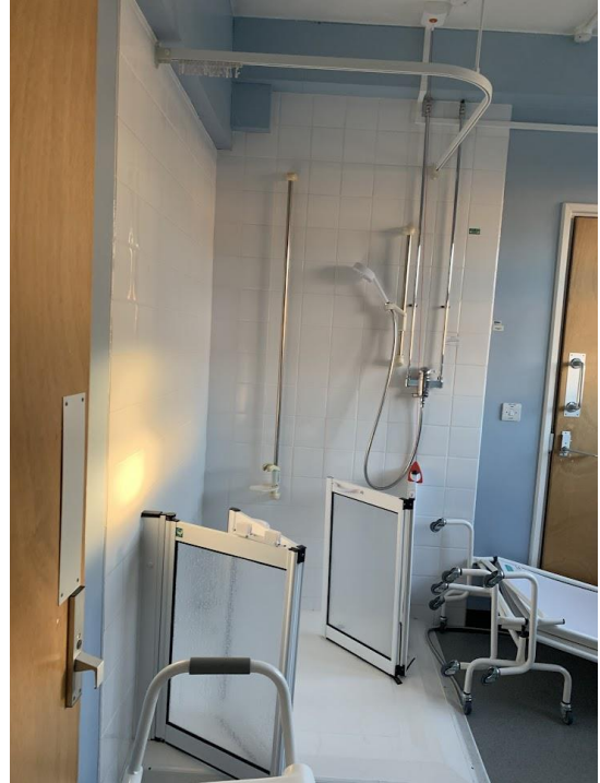
Lack of privacy and dignity with Jack and Jill shower room for both males and females accessed through different doors
