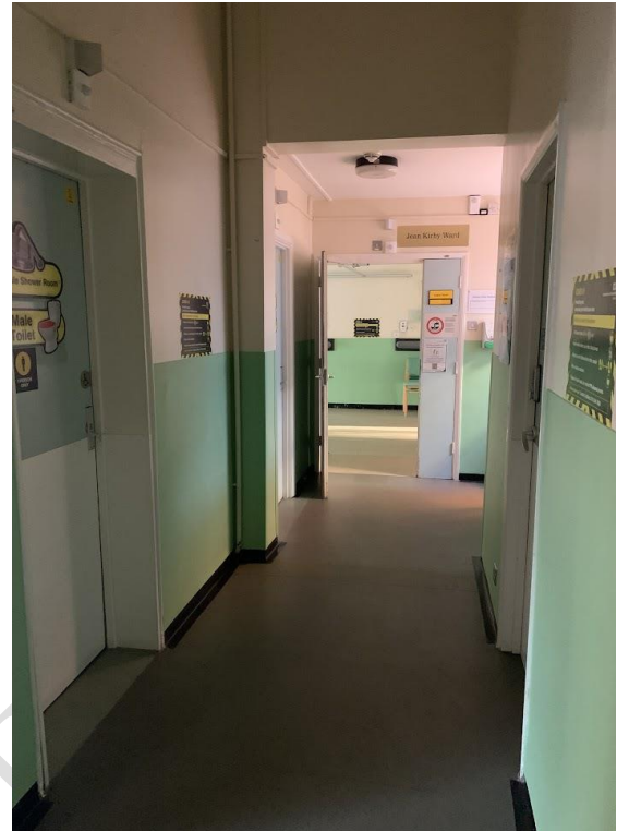
Lack of privacy and dignity - corridor with W.C. shower facilities (male and female)
